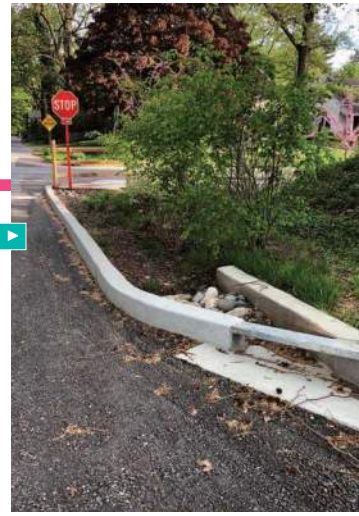
Stormwater bump-out along the street in West Chester Borough, PA.
