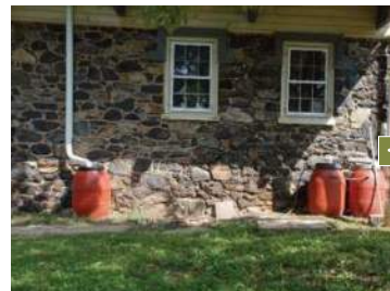
Typical rain barrel downspout connection, private residence.
