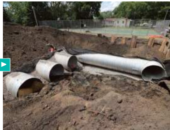
An underground stormwater infiltration system under construction at a park in Minneapolis. (Photo credit: "Infiltration System" by Mississippi WMO is licensed under CC BY-NC 2.0).
