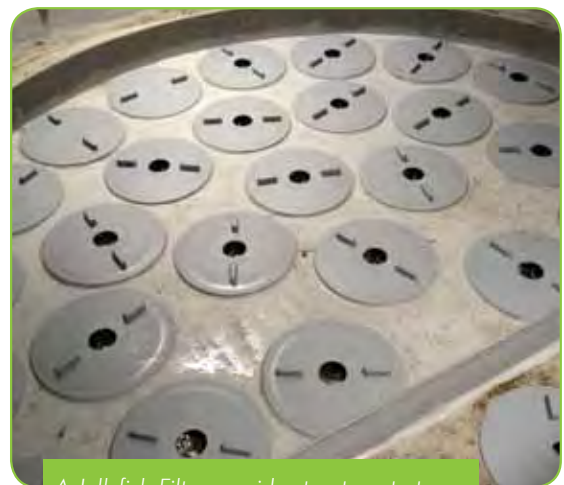
A Jellyfish Filter provides treatment at an Industrial Park in Lake Tahoe, Nevada.
