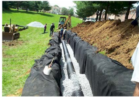
Infiltration trench Chester County, PA
